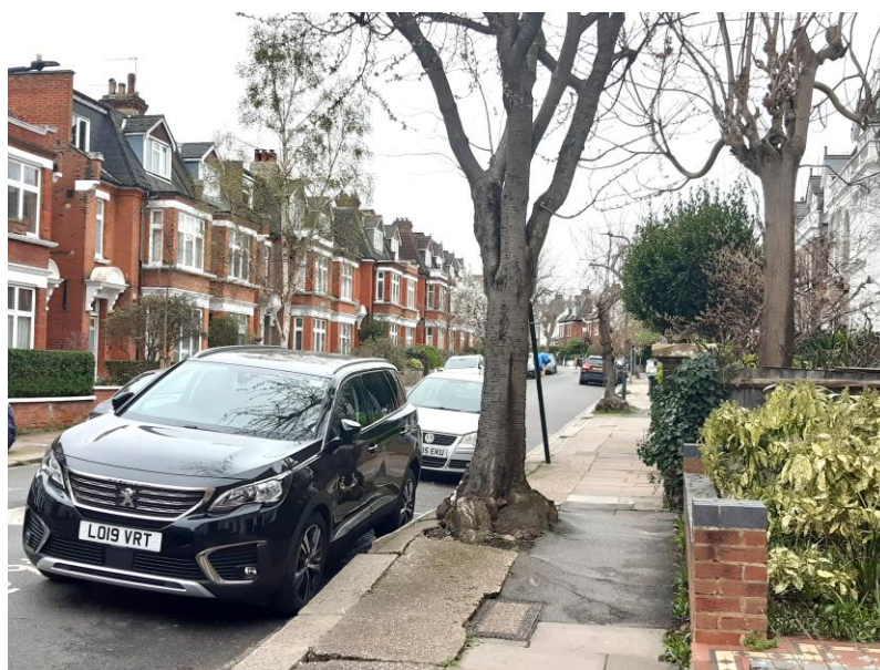
Dyne Road highlighting uneven concrete pavements
